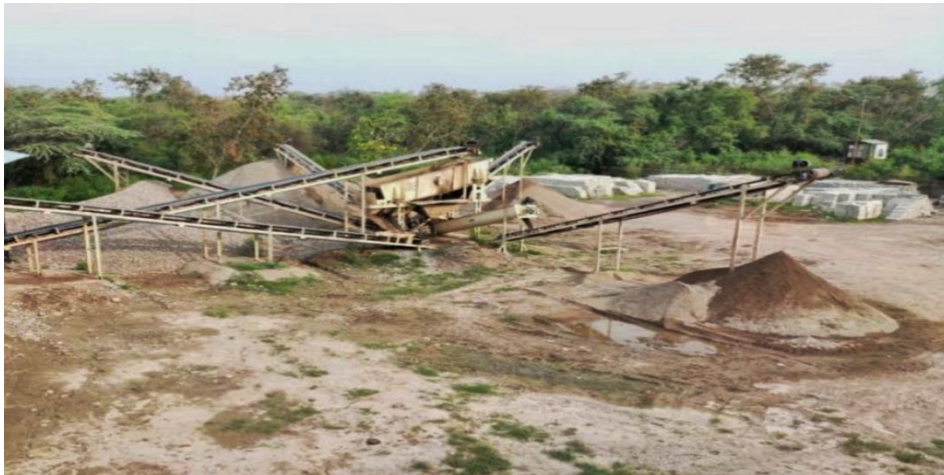
Fig 5 C&D Plant Chandigarh
