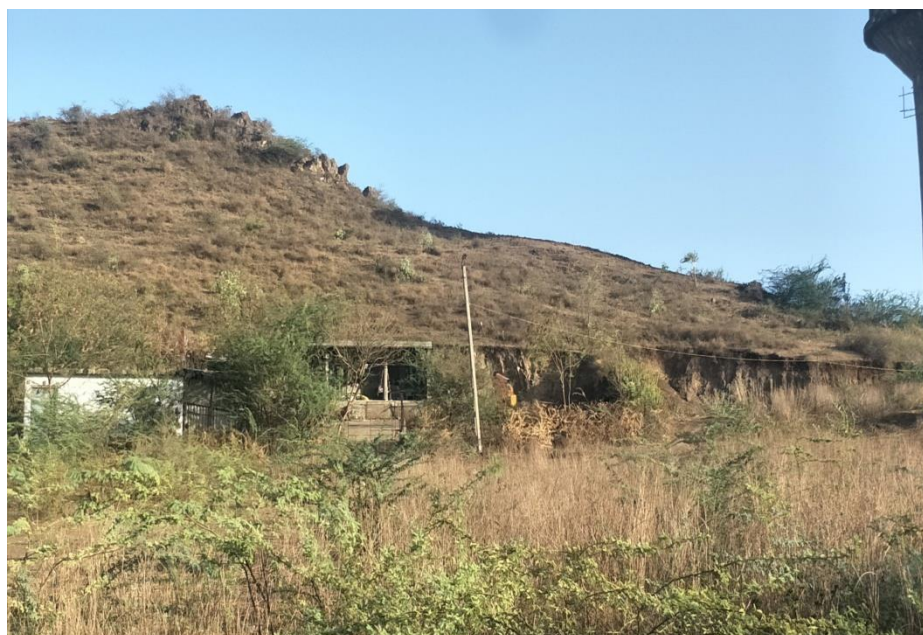
Fig-1. Toe excavation of hill slope at Barman Mota Village of Gujarat
